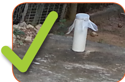
Septic tank ventilation pipe with screen mesh
