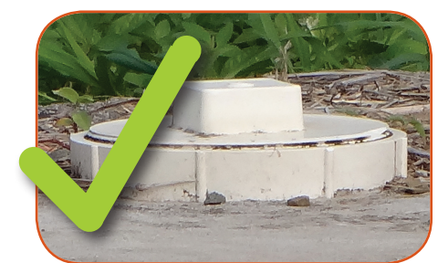
Septic tank sealed with PVC cap
