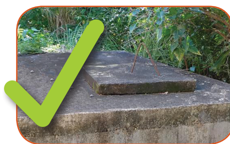
Septic tank with concrete cover
