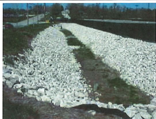
Water detention basins at airports, such as this French-drain system at an eastern USA airport, should be designed to completely drain within 48 hours after the design storm event (photo by R. A. Dolbeer, USDA).
