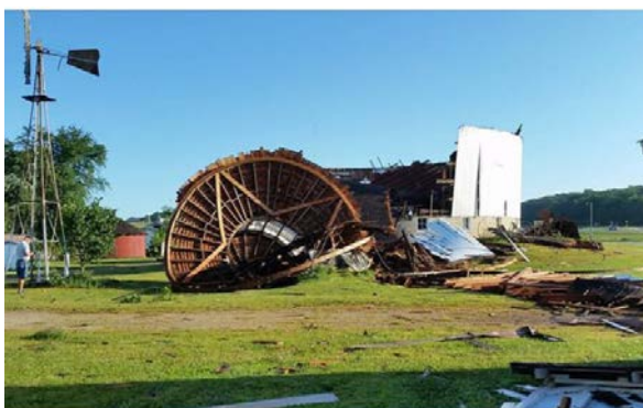
Figure 3-20 Round Barn Damages
