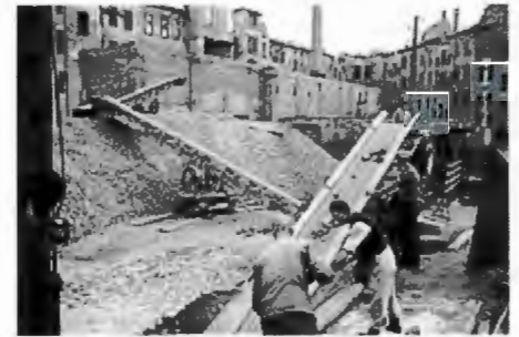
Concrete from a building being sent to a portable crusher. This is the first step to recycling concrete.
